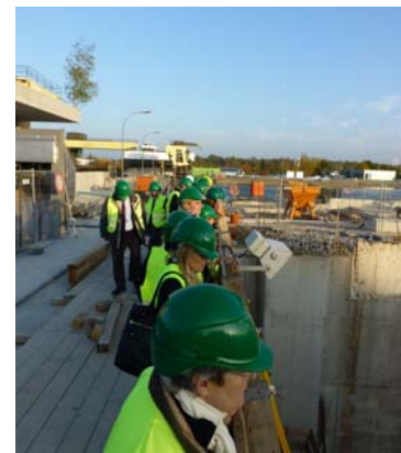
Participants were shown the construction site of the 5th turbine at the Iffezheim Hydropower plant.
