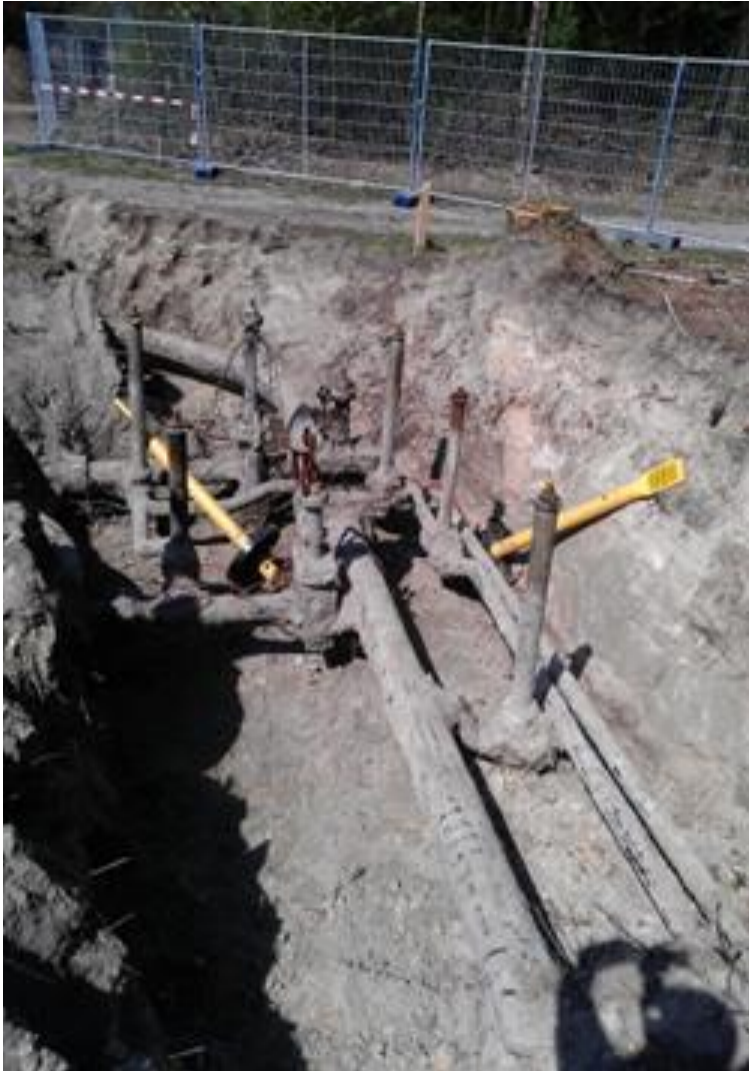
Example of how a difficult to repair leak at a valve station looks like. Source: GIE
